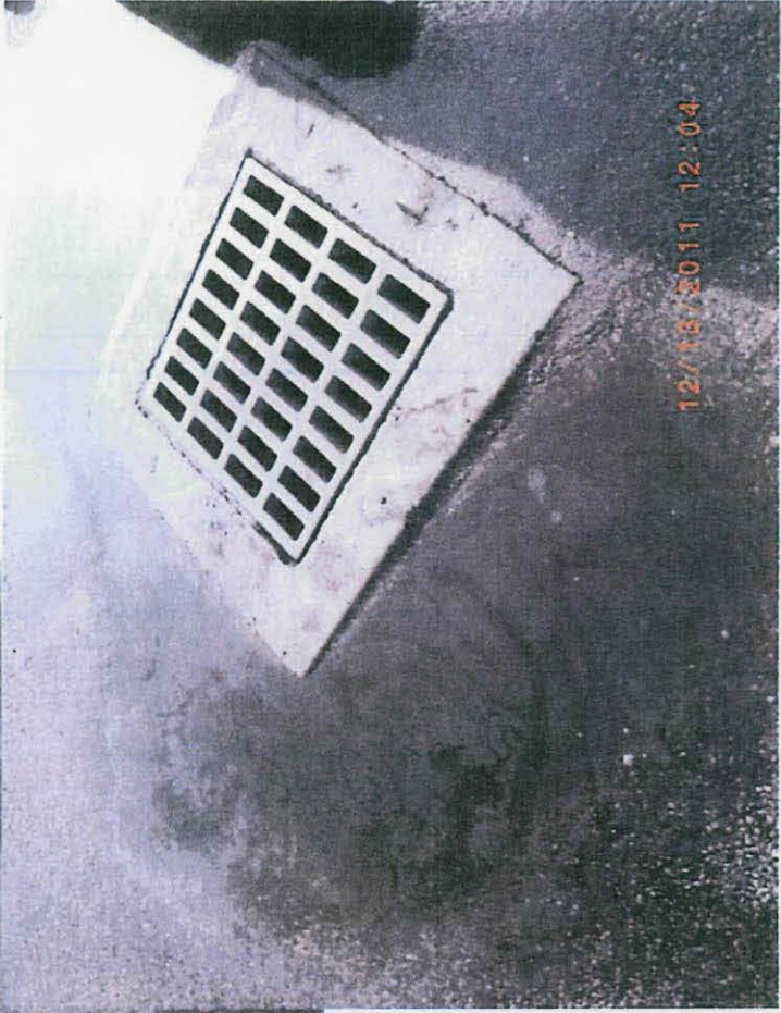
Drop inlet leads directly to receiving stream without treatment, 12-13-11
