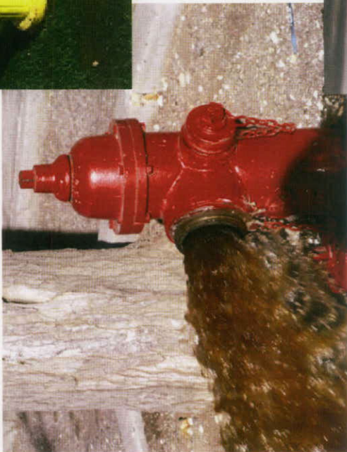
Spot Flushing in Response to BWC
